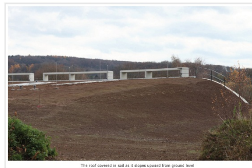
The roof covered in soil as it slopes upward from ground level
